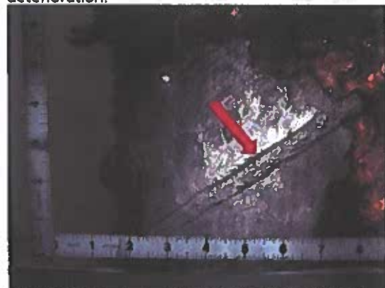
Photo 6: Typical condition of a steel pipe pile below water. Note the missing weld filler material along the spiral weld seam, pile A1 shown.
