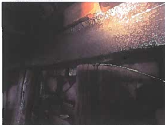
Photo 5: Typical bearing failure at a timber pile, pile E2 shown.
