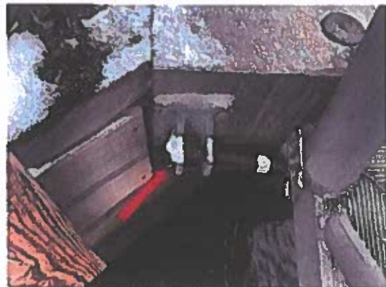
Photo 16: Deformation to the top pin connection of the access gangway. Note the pin is currently only held by the cotter pin.
