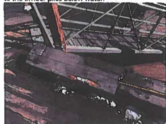
Photo 14: Localized damage to the timber curb located near the floating dock gangway.
