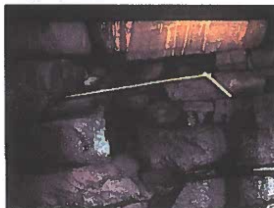
Photo 7: Displaced stone in the quaywall with notable voiding behind, STA 1+42 shown.
