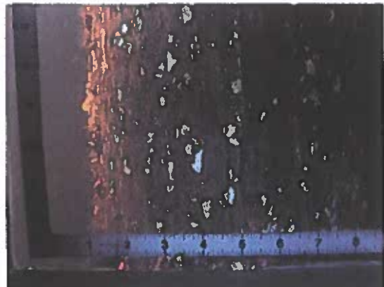
Photo 4: Typical condition of a timber pile below water with notable minor marine borer deterioration.
