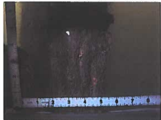
Photo 12: Typical severe marine borer deterioration to the timber piles below water.
