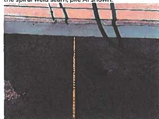
Photo 8: Sinkhole in the asphalt deck, corresponding with voiding in the quaywall below at STA 1+25.
